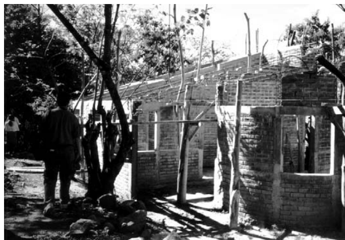
This kindergarten in La Presa is slated to be completed by September.
