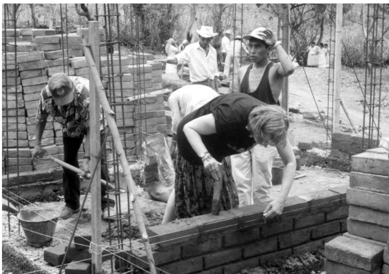
Shirley Novak, laying brick alongside community members to help build the kinder (CIDI-Center for Integral Child Development) in La Estancia, El Salvador, in 1996.
